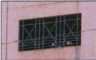
Appropriate: parking garage screening effectively blocks the view of parked cars within the structure.
