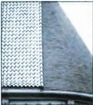
Inappropriate: use of tile and asphalt shingles on the same roof.
