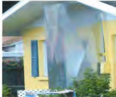
Figure 11: Examples of inappropriately placed utilities, i.e. clearly visible from ground level.
