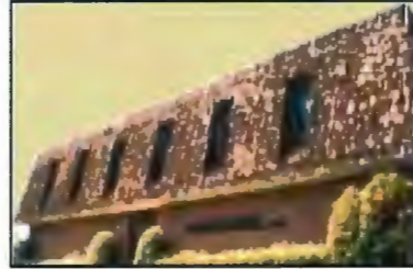
Inappropriate: Cedar shakes and a mansard roof are inappropriate in Downtown.
