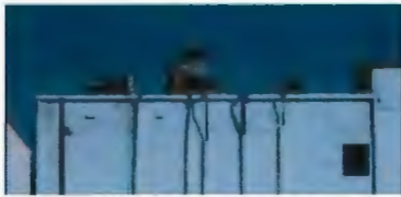
Inappropriate: utilities are clearly visible from the ground located along the edge of the building.
