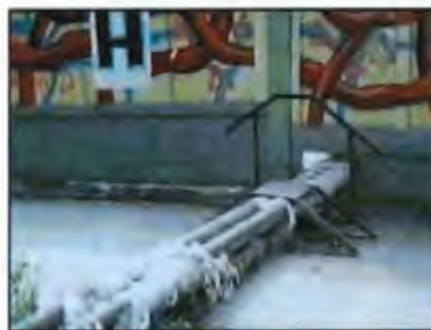
Inappropriate – pedestrian alley is not handicap accessible. among other things.
