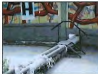
Inappropriate – pedestrian alley is not handicap accessible. among other things.
