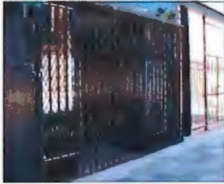
Inappropriate: security gates.
