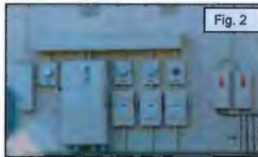
Appropriate: utilities such as gutters, downspouts (fig. 1) and utility boxes (fig. 2) have been painted to match the primary building color.
