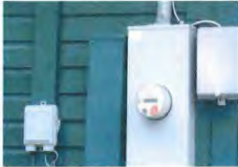
Inappropriate: Boxes should be painted to match the outside of the building.
