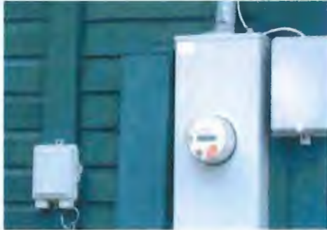
Inappropriate: Boxes should be painted to match the outside of the building.
