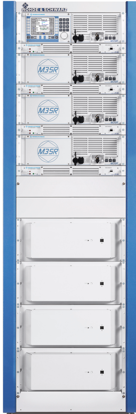
R&S®FU221W4 (VHF) horizontal multicoupler rack installation.
