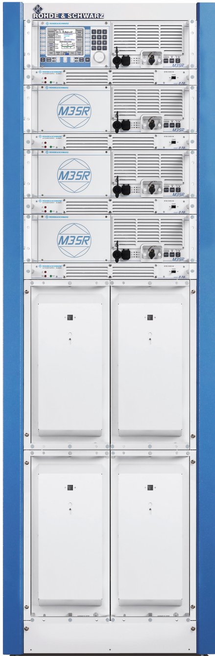
R&S®FD221W4 (UHF) vertical multicoupler rack installation.
