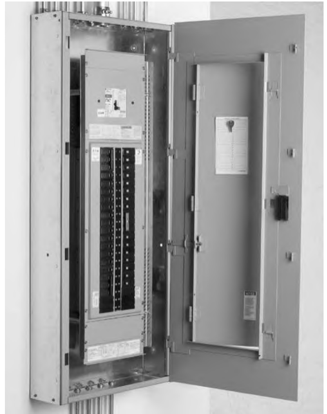
Trim Hanging on Surface Mounted Box
