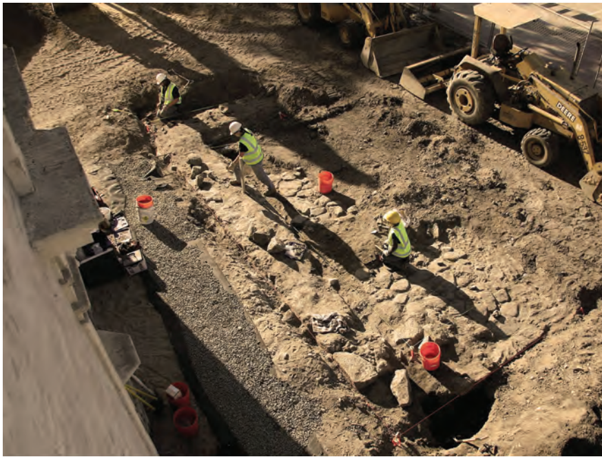
Figure 17. View of the archaeologically-exposed granite foundation footings, boulder pavements, and Roman mortar floorings of the Serra Chapel of 1772. The archaeology field crew, consisting of Gerald Jones, Esther Kenner, and Brenna Wheelis, respectively, are here pictured recovering the granite-boulder pavement of the Serra Chapel of 1772; the footprint of which is located within the forecourt of the San Carlos Cathedral. Photo © Rubén G. Mendoza, 2008.
