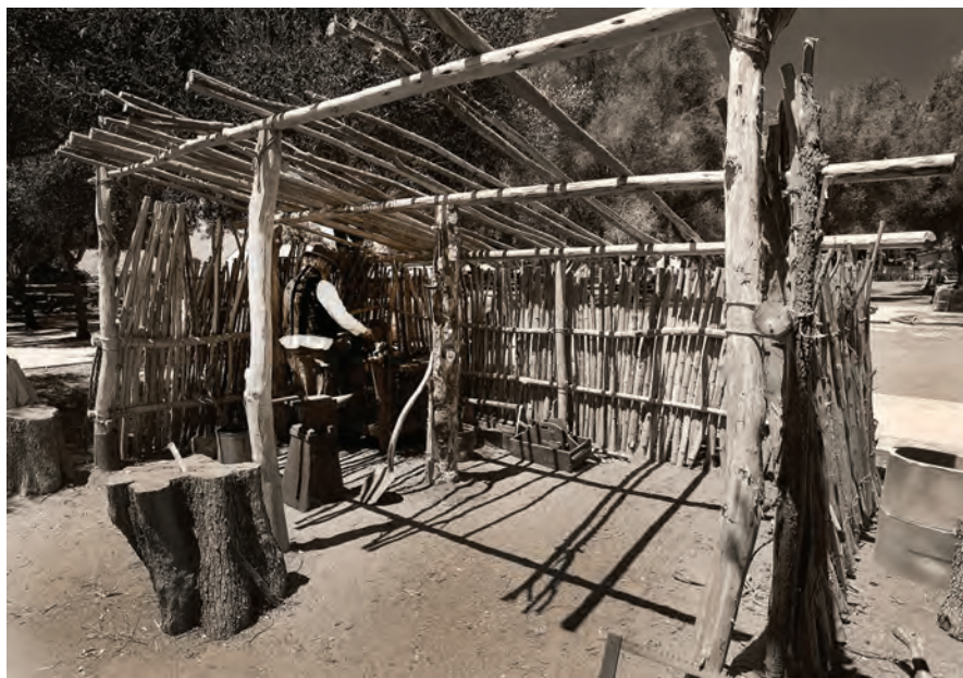
Figure 13. The construction of a jacalon or pole-and-thatch structure was recently undertaken as part of an ongoing restoration and public education effort by the Mission Conservation Program of San Juan Bautista. The structure in question provides an approximation of what one might imagine for some of the earliest structures once located at the Royal Presidio of Monterey. In this instance, construction required the preparation of rawhide straps for use as ties for binding together those poles forming both the perimeter walls and roof of the structure. The effort was directed by program docent and blacksmith John Grafton with the assistance of a host of CSU Monterey Bay student interns. Photo © Rubén G. Mendoza, 2013.
