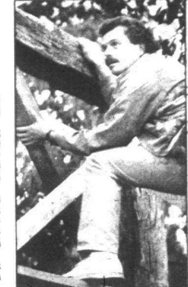
Dean Gilbert sets a brace into place after a crane operator lowers the top beam onto a historic barn Gilbert is reconstructing.
